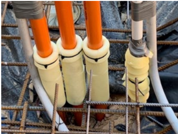
FIGURE 8.6 C GREENZONE® STS applied to 3 orange conduits; GREENZONE® EFTS applied to 1 conduit. Note - 2 grey conduits not treated as they are cast into the slab.
